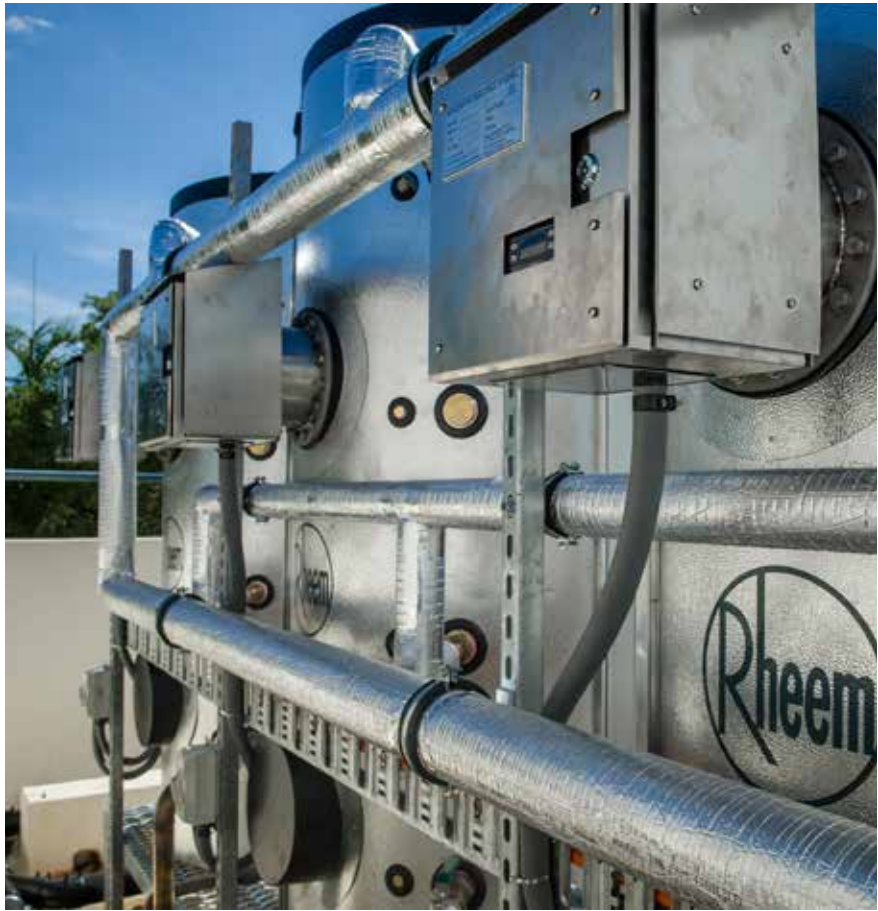
Rheem HS Series solar with electric boosting in the top of solar tanks. Katherine Hospital NT.
